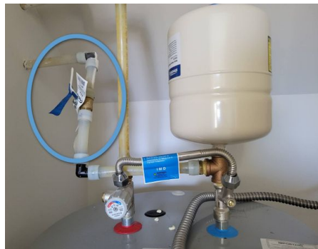
View of water heater water shut-off valve.
