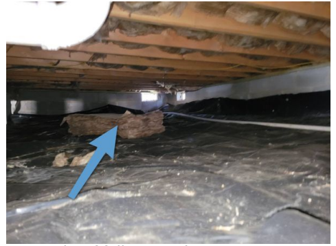
Example of fallen insulation.
