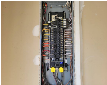
View of electrical panel without cover.
