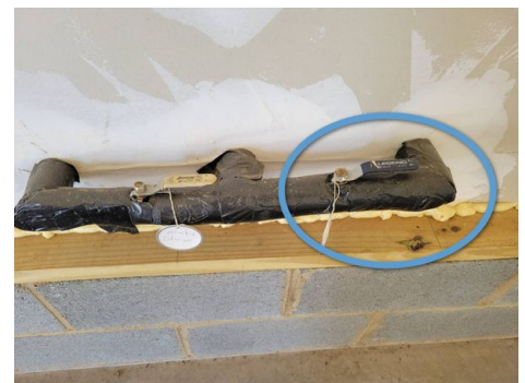
View of main water shut-off valve.
