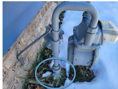
View of main gas shut-off valve.
